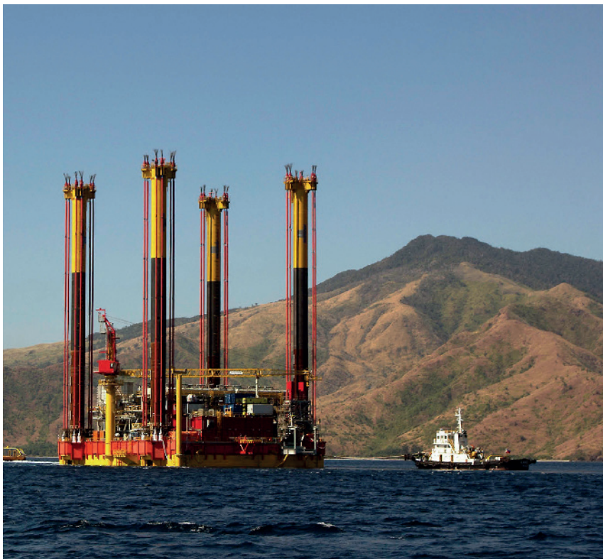
STEADY LIFT: Barge Master used its BM-T700 motion compensating lift system, shown mounted on the deck of Boskalis' Ndeavor , to install the 43-metre bridge.
